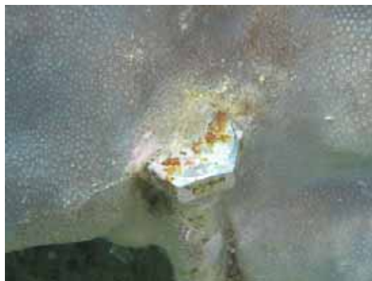
Fig. 6-19 . Coral wrapping around an anchor bolt
